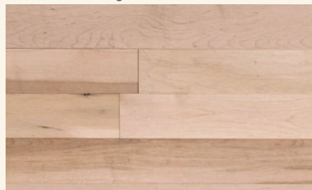
Joints too close together
