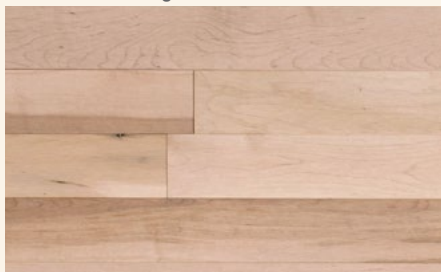
Joints too close together
